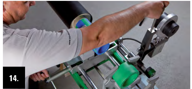
14. After the heating time drive apart the welding machine slide with the crank handle and raise the welding device.
