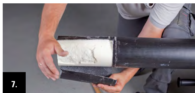
7. Detach the end of the casing pipe and then remove the PUR-insulation layer mechanically on the full skinning length.
