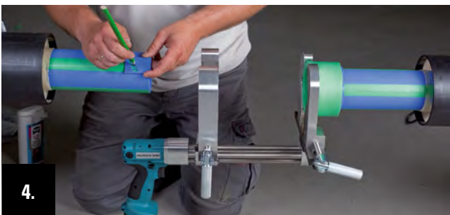
4. The welding depth and the clamping distance are marked by the aquatherm clamping template (blue) in one work.
