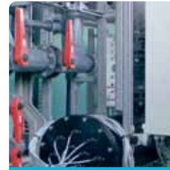
HDPE sea water disinfection
